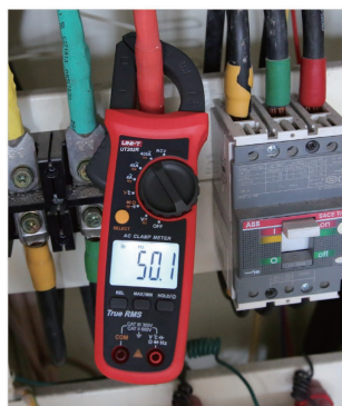
High voltage (600V) frequency measurement
